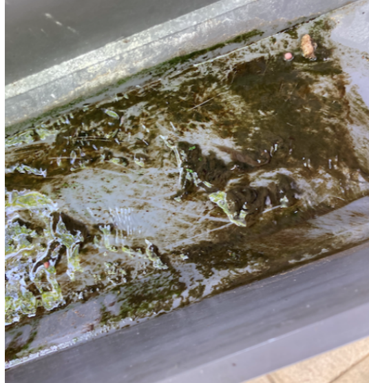
Figure 13. Biomatter in the Pipe System carried by pump. A mix of fish feces, algae and leaves that had fallen in.
